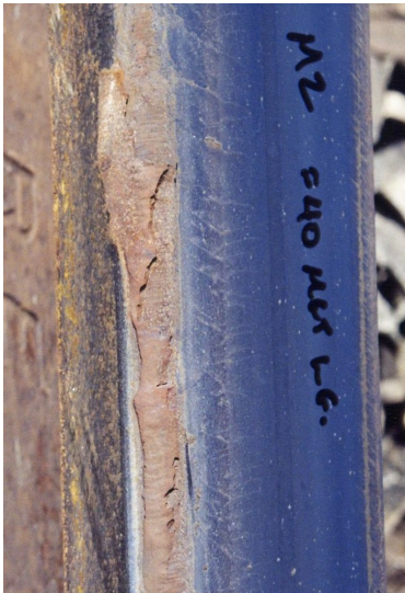
gauge-corner collapse in a dry environment
