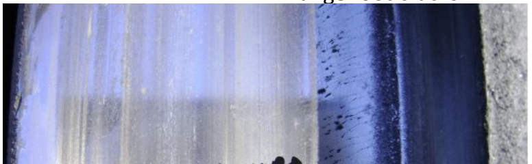
Flange root cracks
