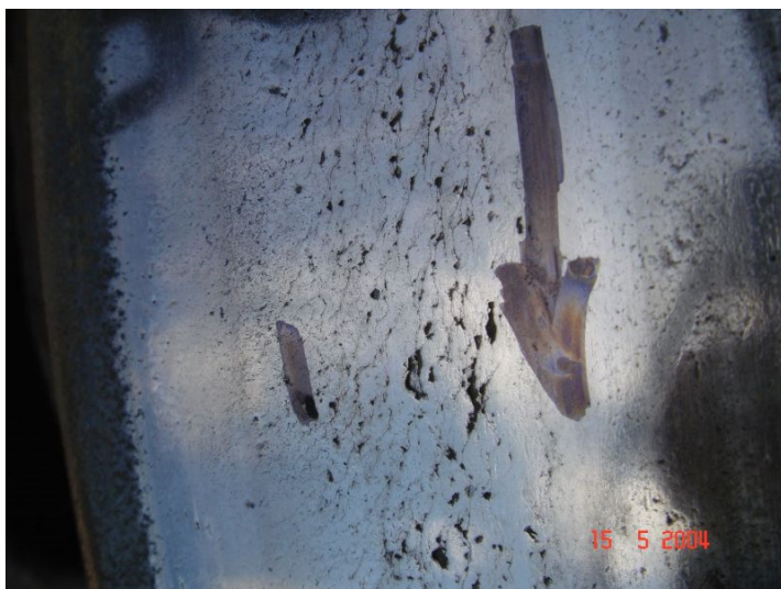
Well-defined cracks on the field/rim side of the wheel.
