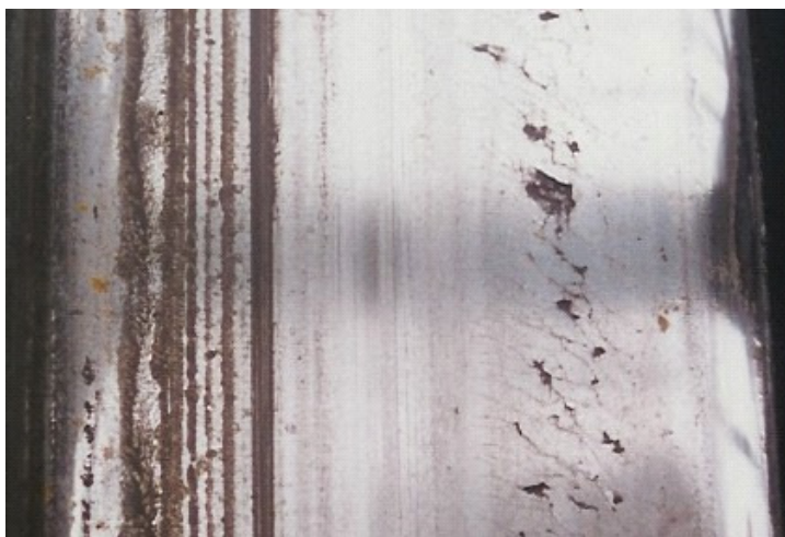
Deeper cracks on the field/rim side of the wheel tread with material starting to shell.
